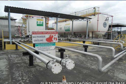
GLP TANKING AND LOADING - JEQUIÉ/BA BASE
